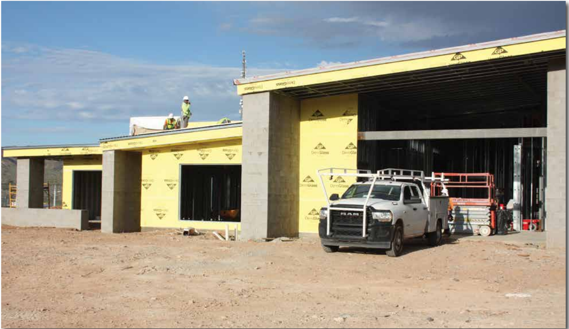
The CV Regional Medical Center new Kearny Clinic building is shaping up.
