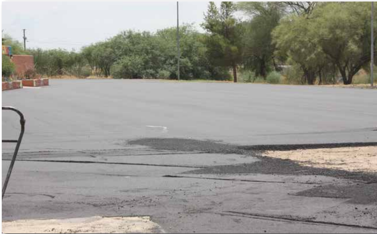
Short Line, the road that's in front of the old Kearny Town Hall and Pool, got a paving job earlier this month. As most people would agree there were lot of holes. But now it's smooth with new asphalt courtesy of Impact Asphalt. Eddie Becerra (left), who owns the company and is a 1983 graduate of Ray District High School, oversees the job. Short Line was paved including new striping from the senior center to Tilbury Drive.
