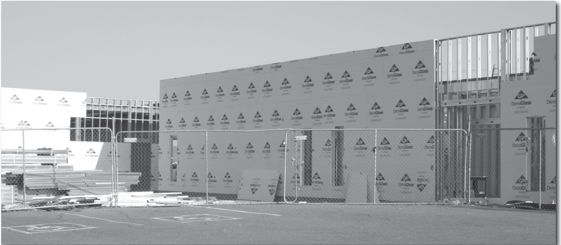
The walls are going up on the new Kearny clinic this week.
