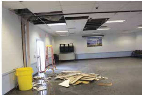
A microburst Thursday left a mess in the San Manuel Community Center as part of the roof was blown away. Nathaniel Lopez | CANP
