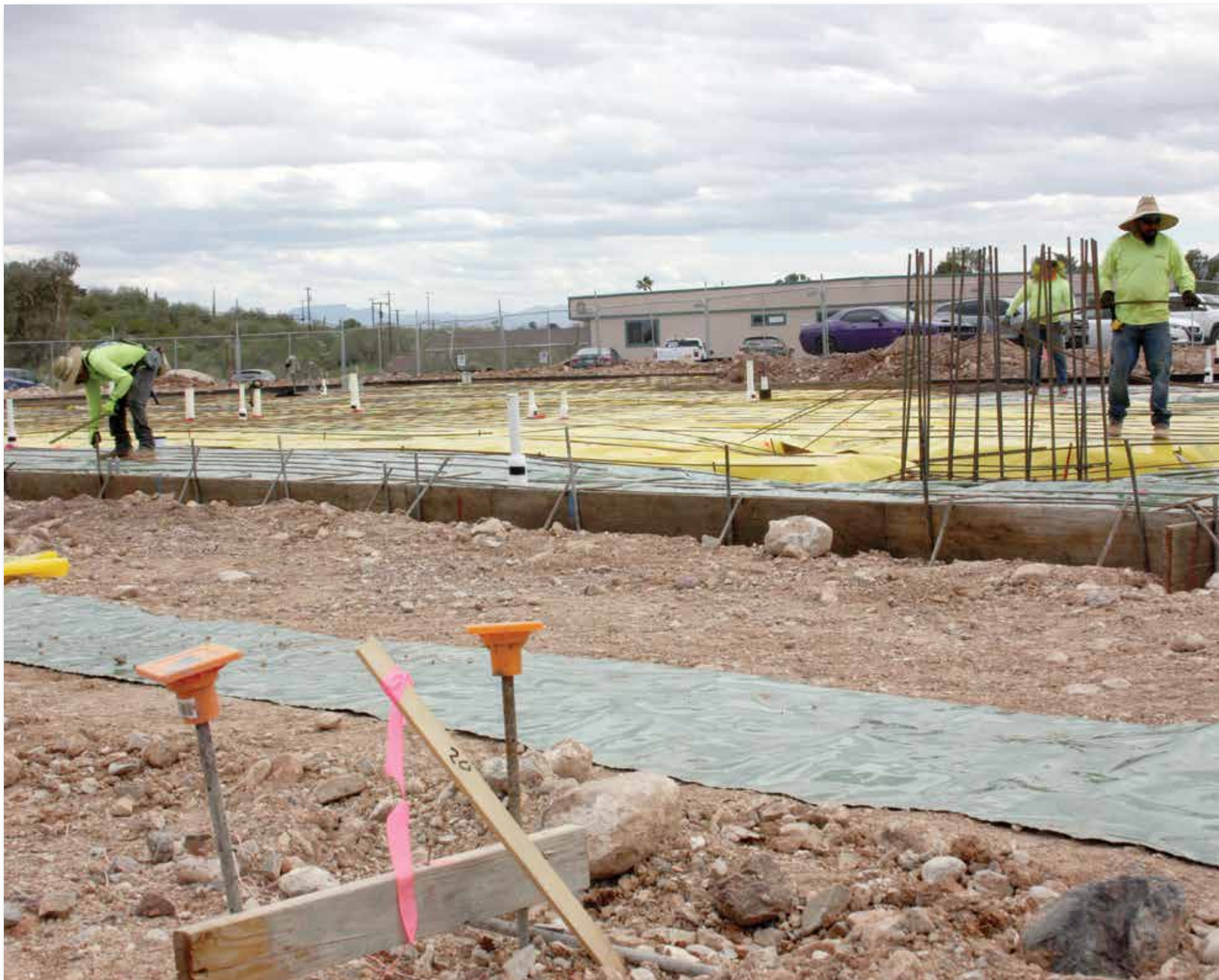
The new Kearny clinic construction continues. Workers install steel to prepare for the concrete foundation to be poured this week.
