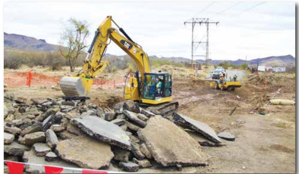
Demolition on the Panther Drive Queen Creek Bridge – making way for the new bridge. Debbie Torres | CANP
