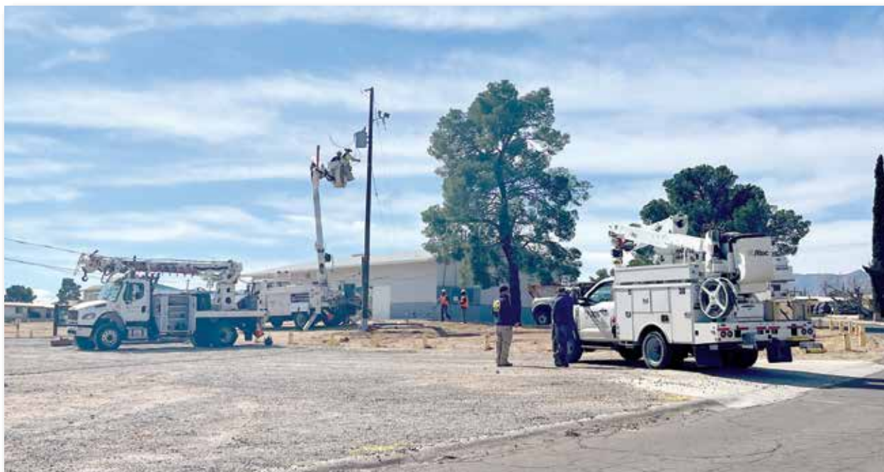
APS crews and contractors working on power lines and replacing light poles at the San Manuel Community Center and City Park. T.C. Brown | CANP
