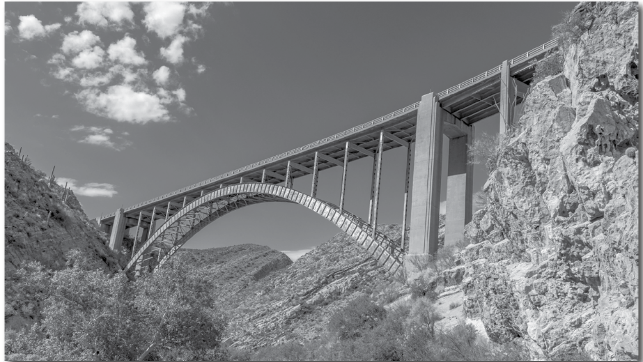
This aging bridge east of Superior will be replaced. Construction begins soon.
