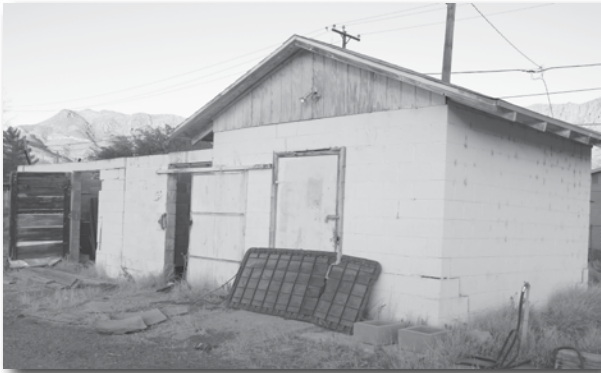
Structure planned to be demolished and replaced with restrooms. Nathaniel Lopez | CANP
