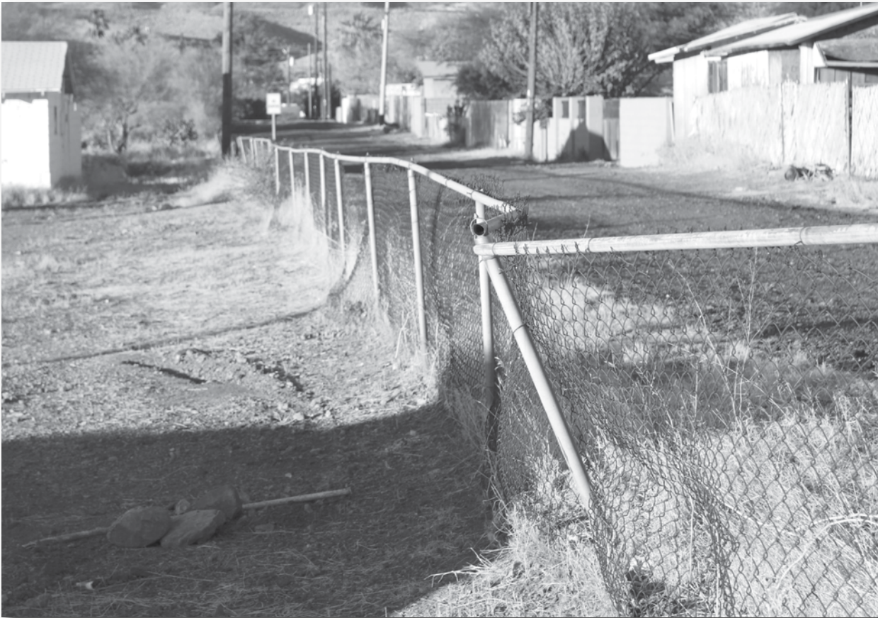
Most of the fence surrounding the Fairview Cemetery is broken, or completely falling apart.
