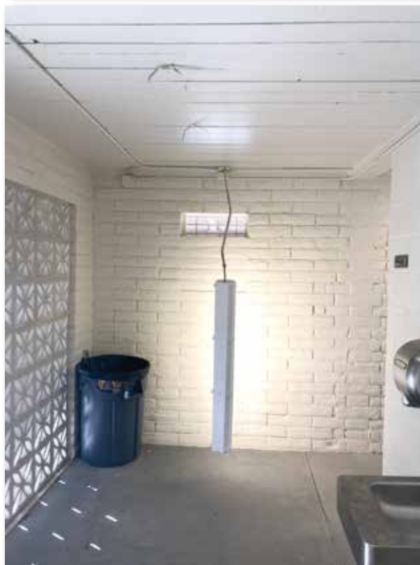
Vandals tore down lights and ripped a sink off the wall at the newly renovated restrooms at the Oracle Park.
